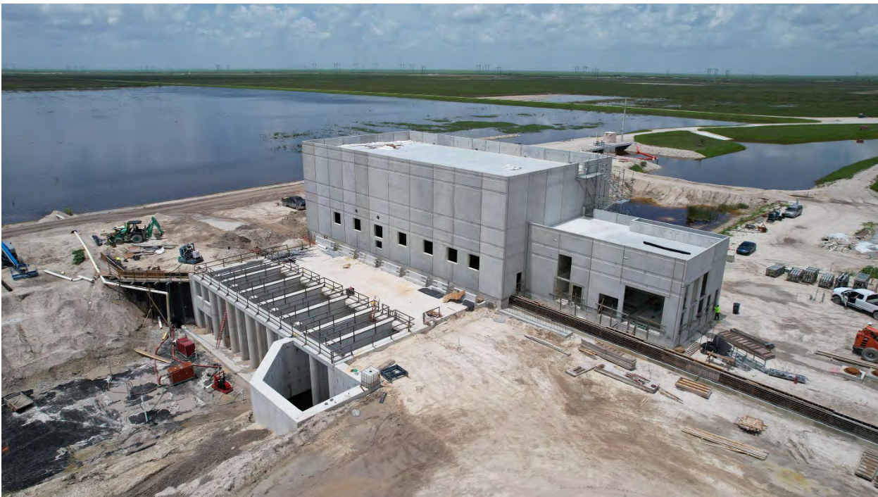
STA -1W Expansion # 2: Image shows ongoing construction activity at G-781 Pump Station
